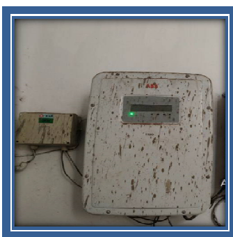
Grid Connections on the rooftop Of A.J.C. Bhawan (Science Building)
