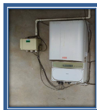
Grid connections on the rooftop of K.M. Hall
