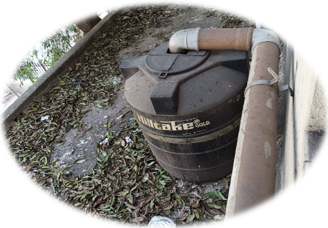
Fig. 2 : Rain water Harvesting Tank
