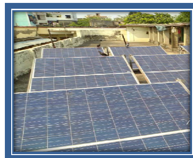
Solar panel on the rooftop of K.M. Hall
