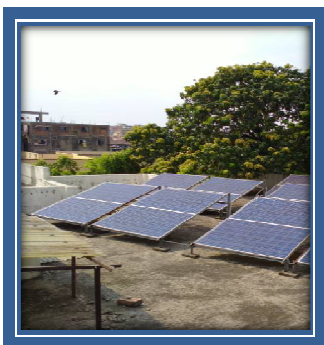
Solar panel on the rooftop Of A.J.C. Bhawan (Science Building)
